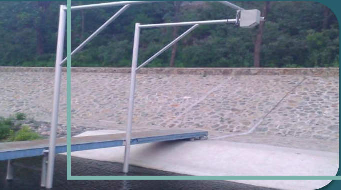
Non-contact discharge measurement (RQ-30) for the sponge city project, Beijing 非接触式流量测量 (RQ流量计)，北京海绵城市雨洪工程
